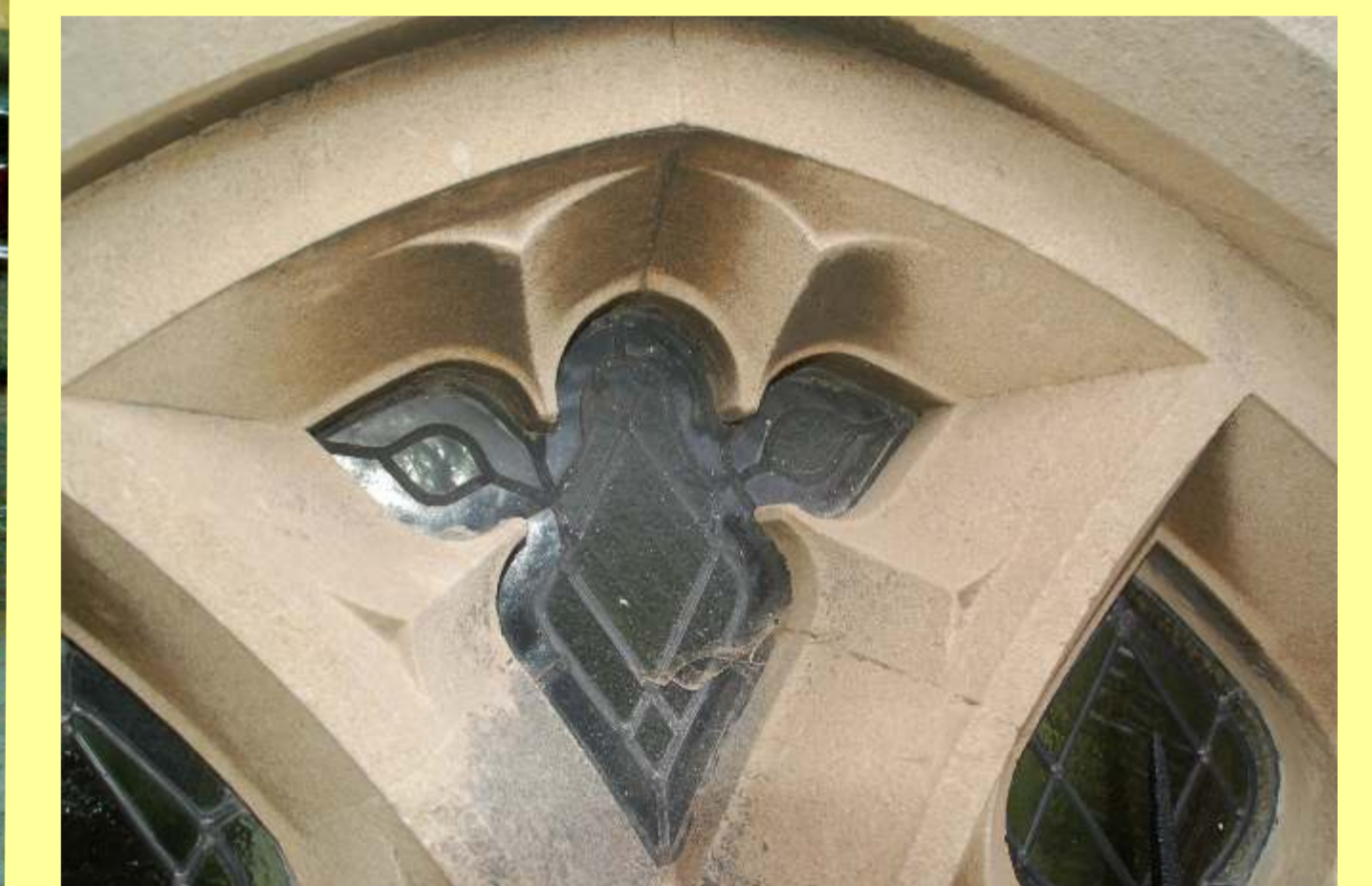
The stonework frames were repaired with new carving on much of the detail.
